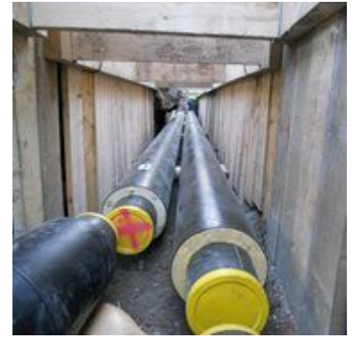
Illustration 5 CDHN under ground pre-insulated pipe work
